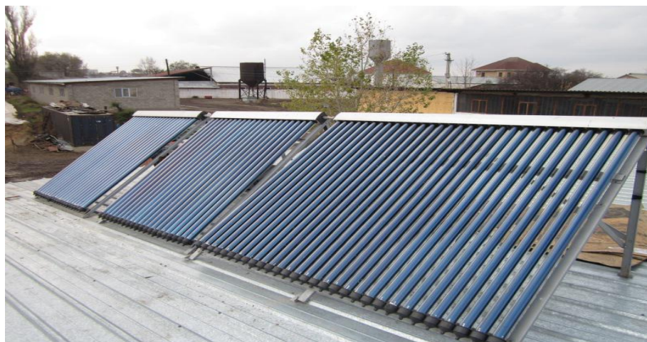
Figure 2. General View of Solar Water Heating Unit
